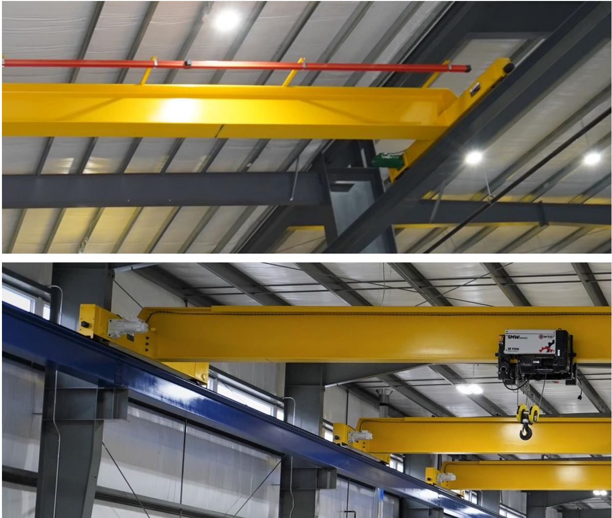
1.1 STT End Trucks on a Bridge Crane
