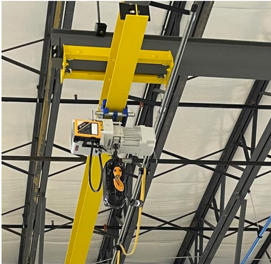
2.2.1 SBK End Truck Part of a Crane System
