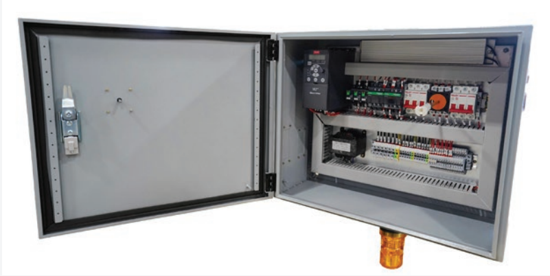
VFD Control Panel with Amber Strobe Light
