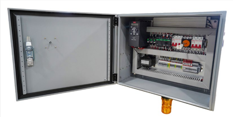
VFD Control Panel with Amber Strobe Light
