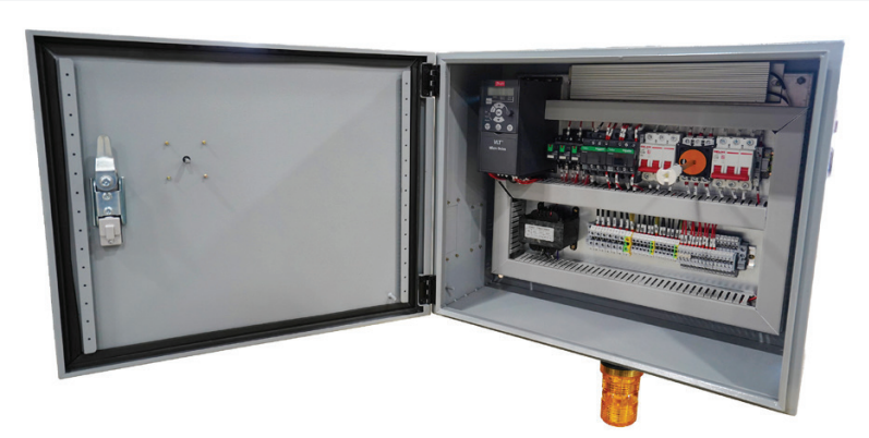
VFD Control Panel with Amber Strobe Light
