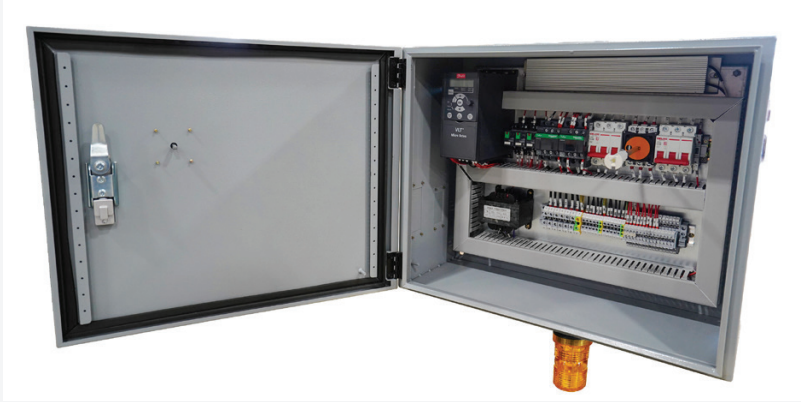
VFD Control Panel with Amber Strobe Light
