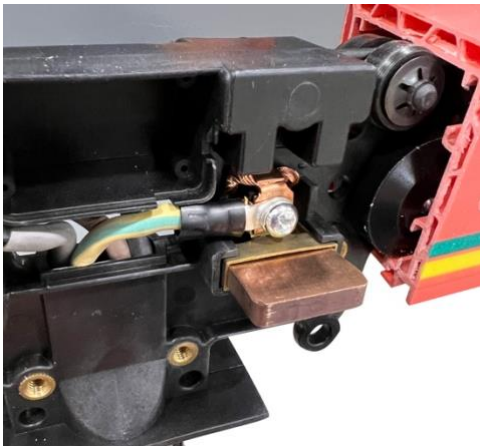
4.6.9 40 Amp Single Collector Installed
